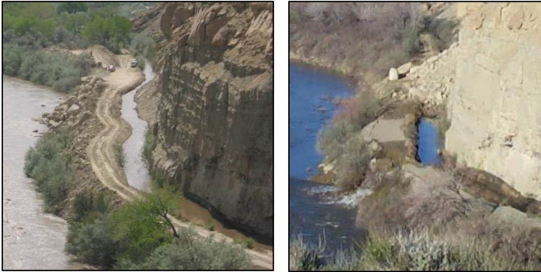
Figure 6-108 Landslide Occurrence at Farmers Mutual Ditch in Preparedness Area 4
