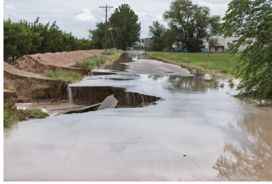
3: Flood waters erode major roadway in rural community (Las Cruces Sun News)
