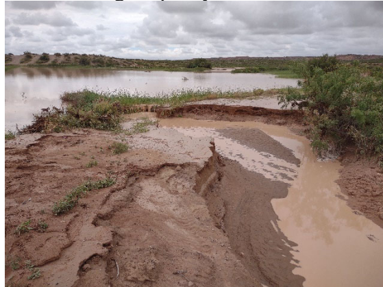
1: Erosion and flooding along the La Union B dam
